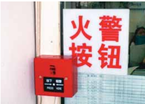
Warning devices at the SNFC plant
