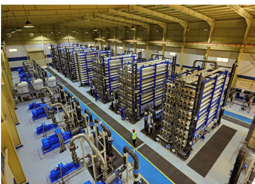
Al Yosr Desalination Facility, Egypt
