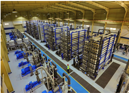
Al Yosr Desalination Facility, Egypt
