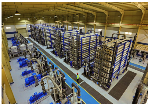
Al Yosr Desalination Facility, Egypt
