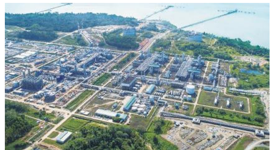
Two existing LNG trains and an expanded train under construction, LNG tanks, jetty, etc.
