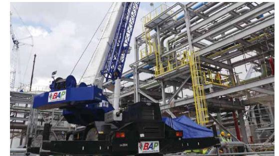
Industrial Machinery Division (Nikken Corporation)
