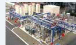
Dehydrogenation plant in Kawasaki City
