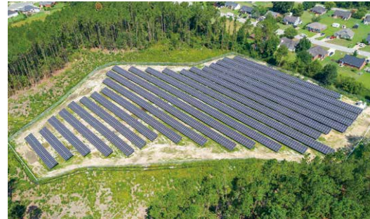
MC Energies Corporation (Diamond Generating Corporation)
